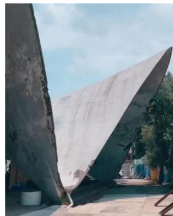
Figure 7. It is worth noting that after the 2017 earthquake (one of the strongest recorded in Mexico City) Los manantiales suffered minimal damage, demonstrating the structural efficiency of this type of structures.
