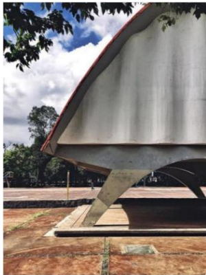
Figure 5. Front view of the cosmic ray pavilion, which is made up of a reinforced concrete shell, a side wall in concrete waves and the pavilion's foundation.
