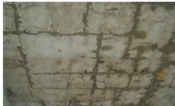
Fig. 1 heat of hydration leads to cracks
