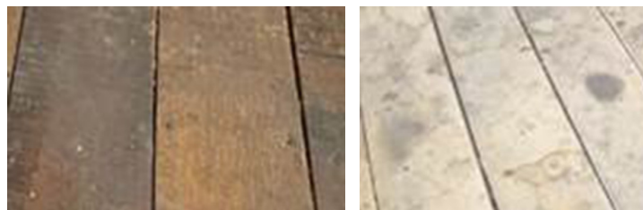
Figure 6. Floor condition of UPR 1 (left) dan UPR 2 (right).
