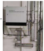
图12 GAS DETECTOR ( IN GAS DETECTION SAMPLING PANEL )
